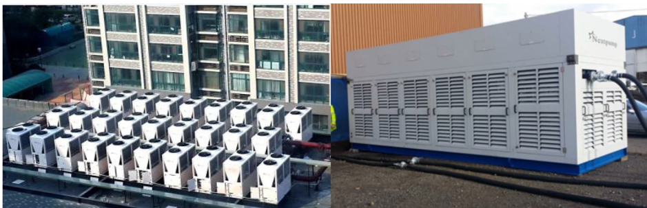
Figure 15-13: Large capacity ASHP installation examples: Rooftop installation (left) or ground level installation (right, unit shown is 700kW in size and 8m in length, image courtesy of Star Refrigeration).
