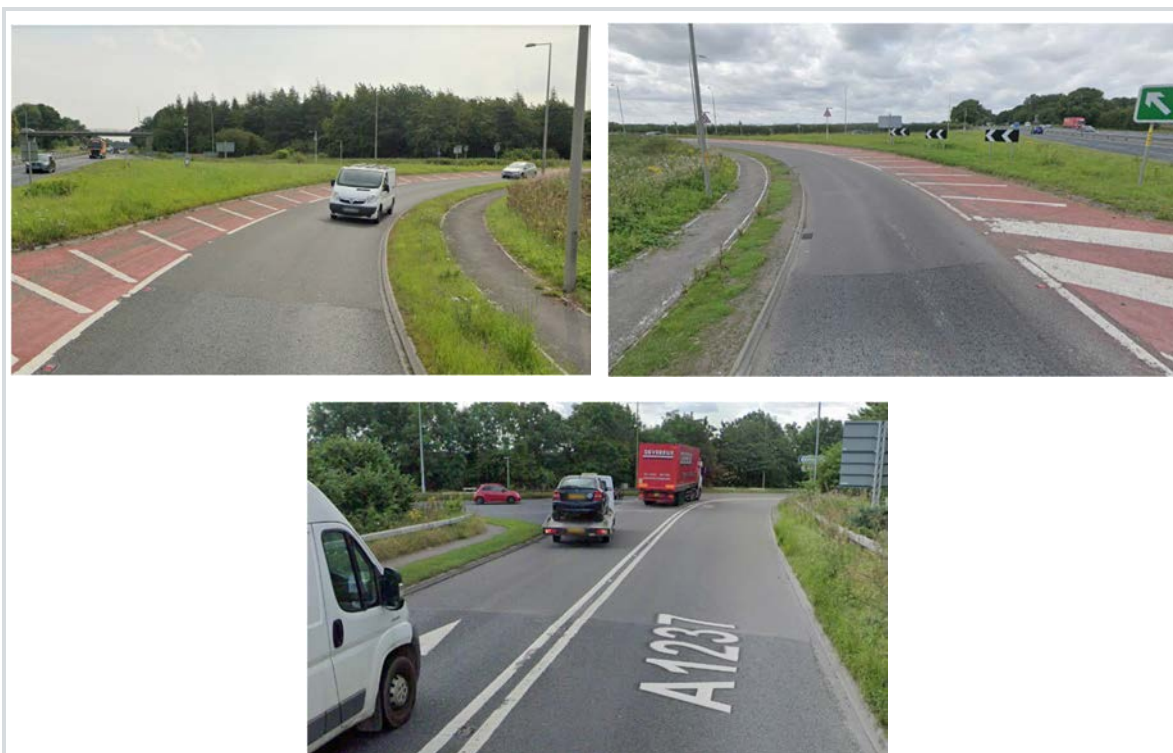
Figure 11. A64 Material A start and end joints
