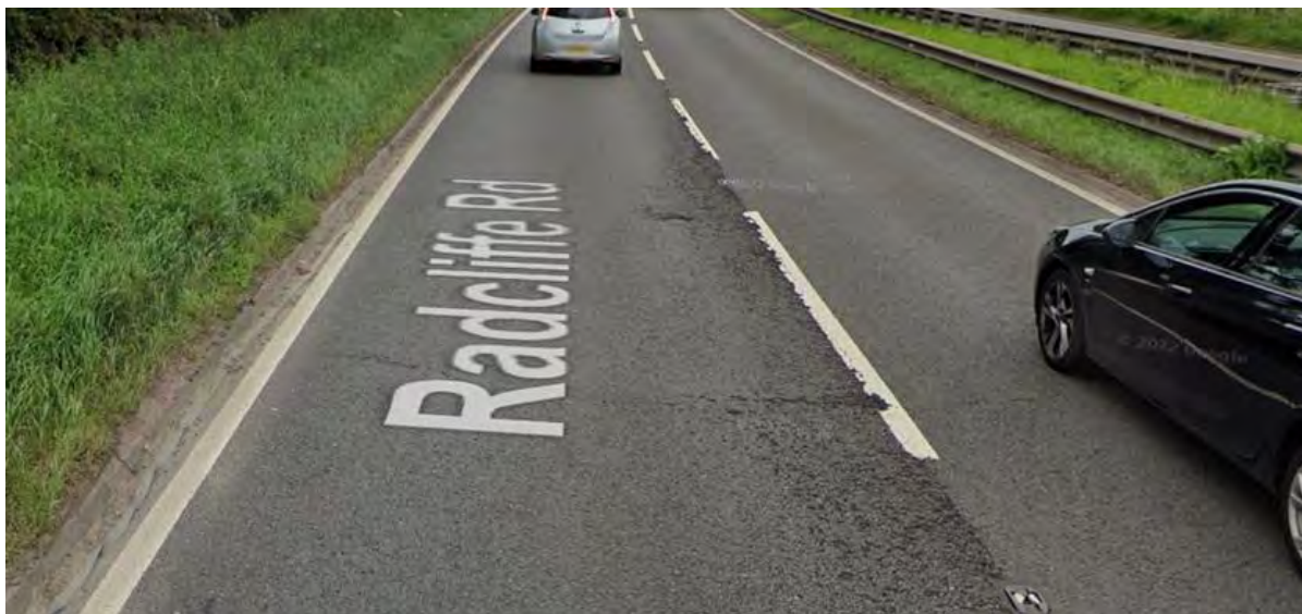
Figure 3.5 - A52 Stragglethorpe Rd to Nottingham Rd transverse cracking and raveling
