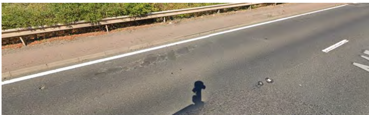
Figure 3.9 - A45 Ryton-on-Dunsmore apparent structural deterioration (Google Street View, 2018)
