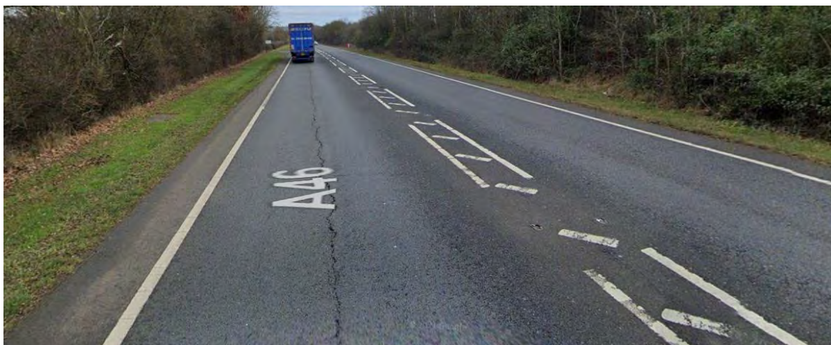
Figure 3.6 - A46 Stratford-upon-Avon Bypass longitudinal cracking from underlying HBM joints
