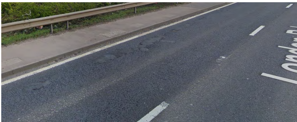
Figure 3.8 - A45 Ryton-on-Dunsmore apparent structural deterioration (Google Street View, 2018)
