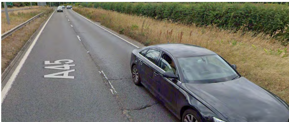
Figure 3.10 - A45 Ryton-on-Dunsmore significant transverse cracking (Google Street View, 2022)
